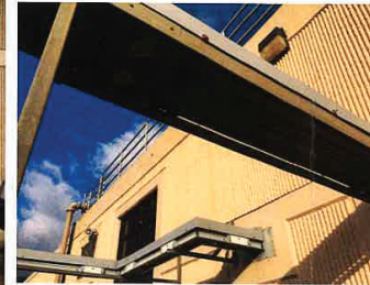
2000AMP SERVICE ENTRANCE BUSWAY
