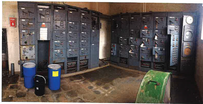
ABANDONED AND DE-ENERGIZED MCC
