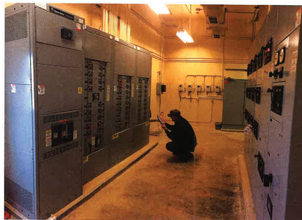
SWITCH BOARD 101 AND MCC-101
