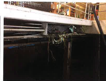
TYPICAL JUNCTION BOXES OPEN
