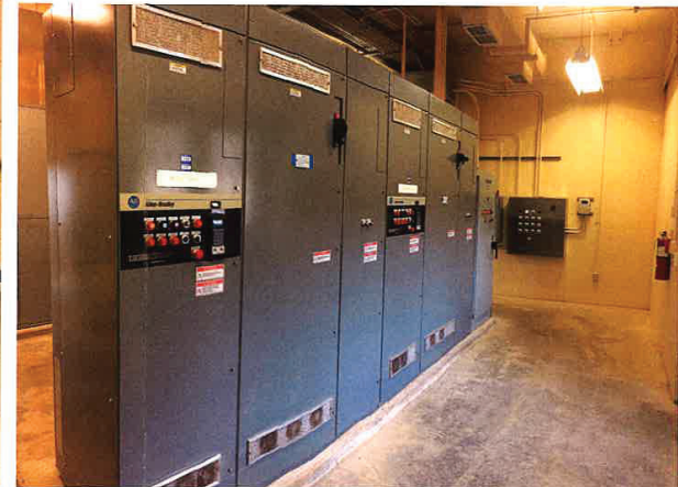
CUSTOM VFD PANELS
