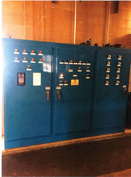
CUSTOM FILTER CONTROL PANEL
