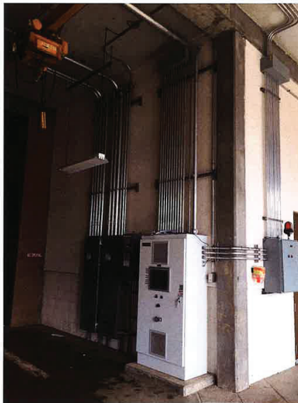
DP-2, DP-3 & REMOTE I/O PANEL FP-08-01
