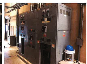
SWITCHBOARD AB-1, AB-2 & TIE BREAKER
