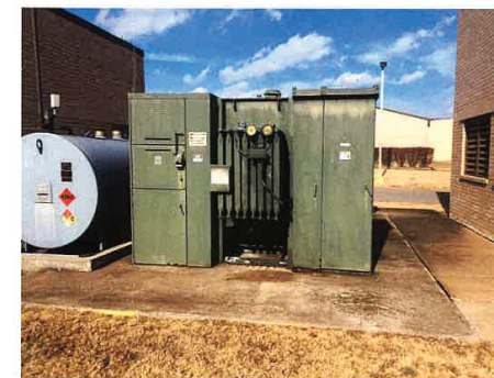
TRANSFORMER & SWITCHES PI-2
