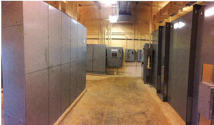
BACK OF MCC-101 AND CUSTOM VFD PANELS
