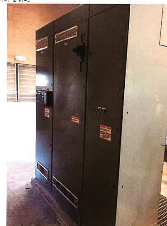
NEVER ALLEN BRADLEY CUSTOM PANEL FOR RW-P-1-1 INFLUENT PUMP
