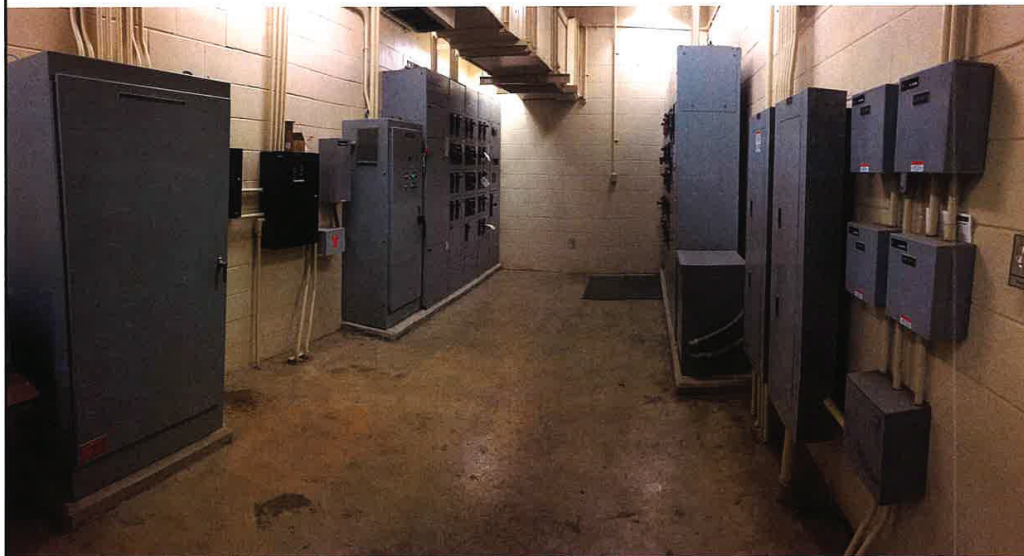
SOLIDS DEWATERING BUILDING ELECTRICAL ROOM
