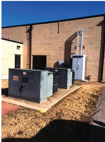
TRANSFORMER NO. 1, NO. 2 & DP-1
