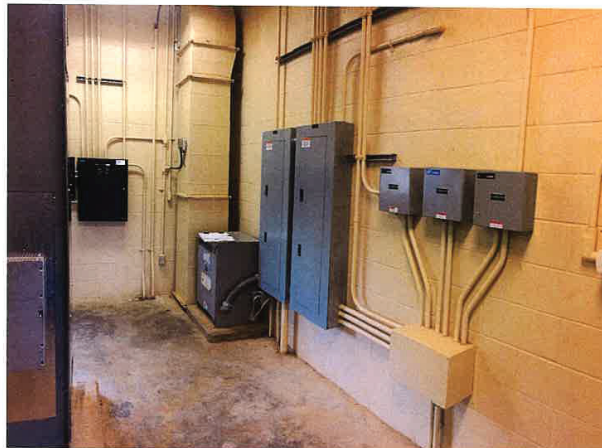
LIGHTING PANELS, TRANSFORMER AND FIRE ALARM PANEL
