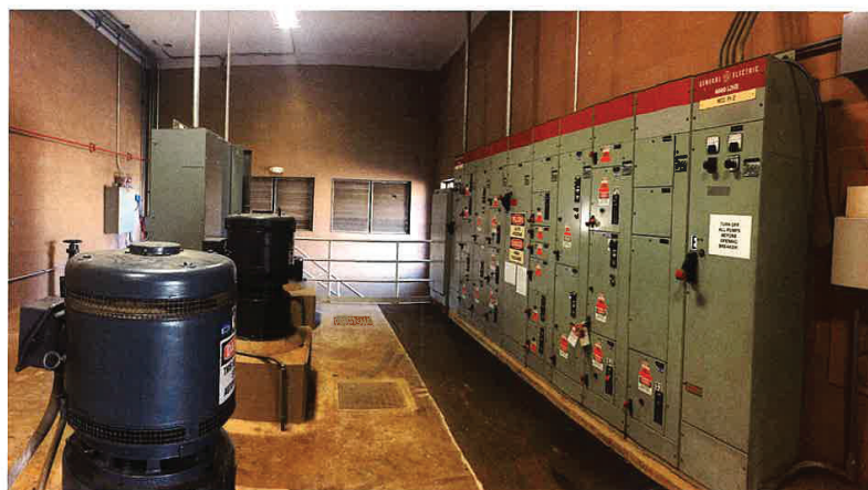
MCC PI-1 & PI-2 GE MOTOR CONTROL CENTERS
