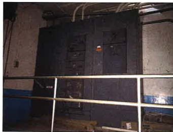
LABELS MISSING OR UNKNOWN SQUARE-D SAFLEX SWITCHBOARD
