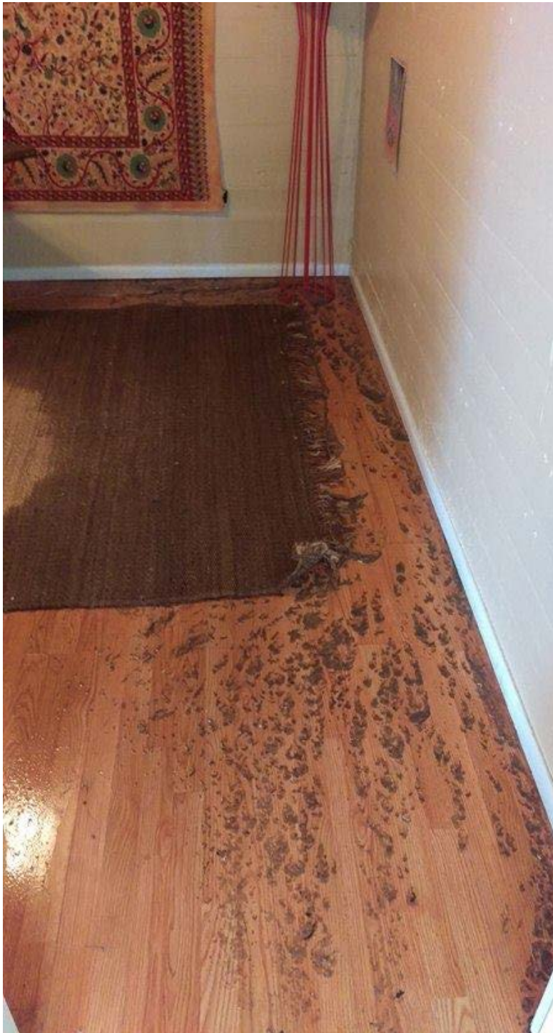
Damages pictured in photo: burlap rug in office
