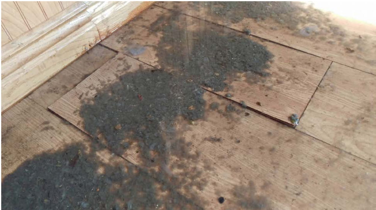
Worst hit bedroom. Where roommates "X" and "Y" live. They had about 10" of standing water before shut off.
