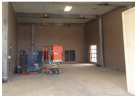
Old chlorine storage area ready for ozone.
