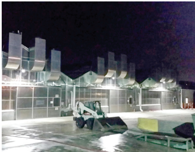
LED lights in use at solar drying houses on BMS.
