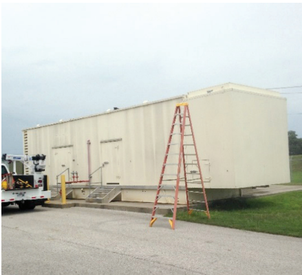
Two megawatt generator at the West Side WRRF.
