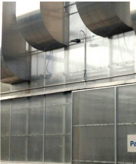
Downturn LED lights installed at BMS.
