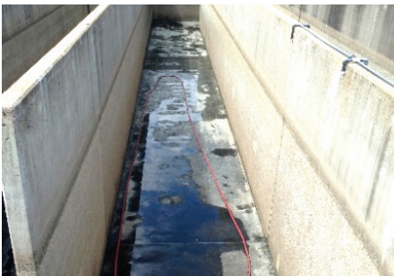
South basin ready for ozone equipment.
