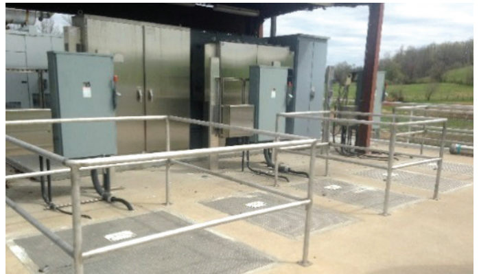
New safety rails at Farmington Lift Station (LS 12).
