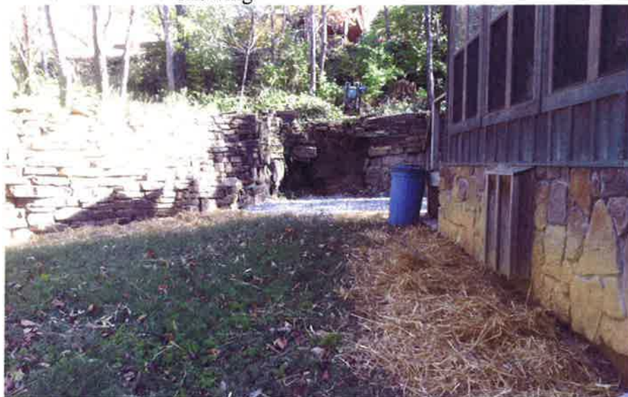
Damaged and Undamaged Wall Sections
