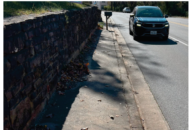
Off-camber sidewalk with no buffer & wall
