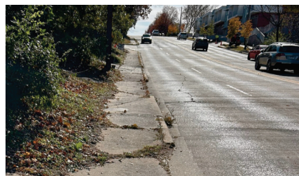
Cracked & uneven surfaces in both the roadway & sidewalk
