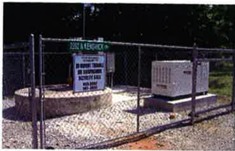
Lift Station #39 – 2393 N. Kenswick
