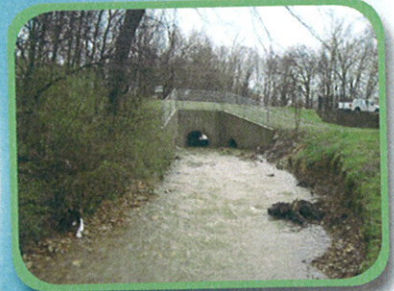
flood waters and streambank erosion
