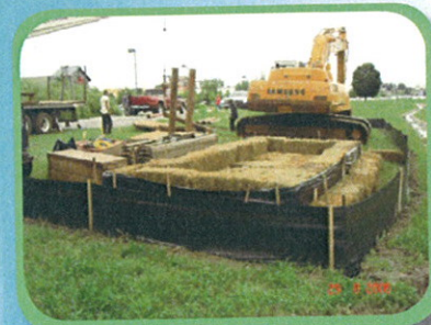
sediment filter used during construction
