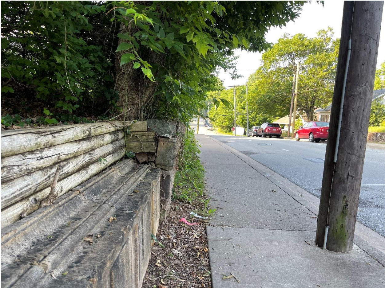
Looking south, the existing tree near the shared property line between 216 and 212 appears to be pushing the top of the wall out, causing it to lean toward the sidewalk.
