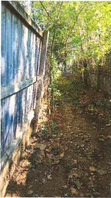
Shows the fence being on top of garden beams
