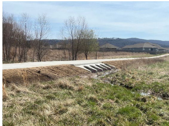
Picture 12: Woolsey Trail Culverts
