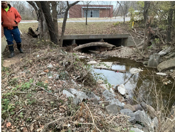
Picture 1: North St. & Scull Creek Before
