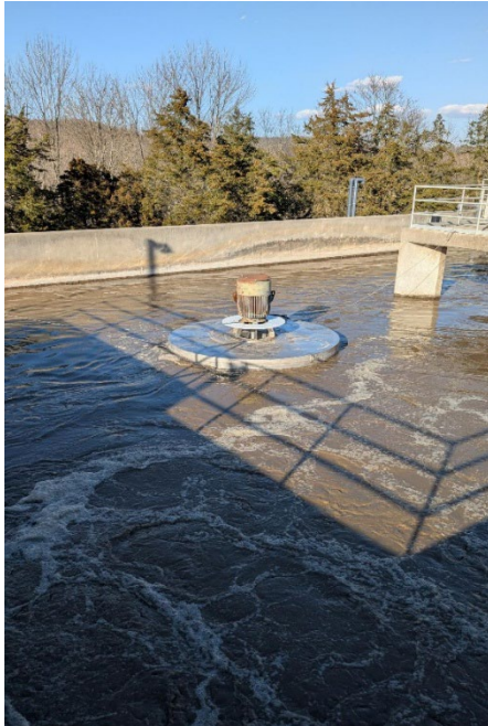
*Pictured above, floating aerator just before being put into service
