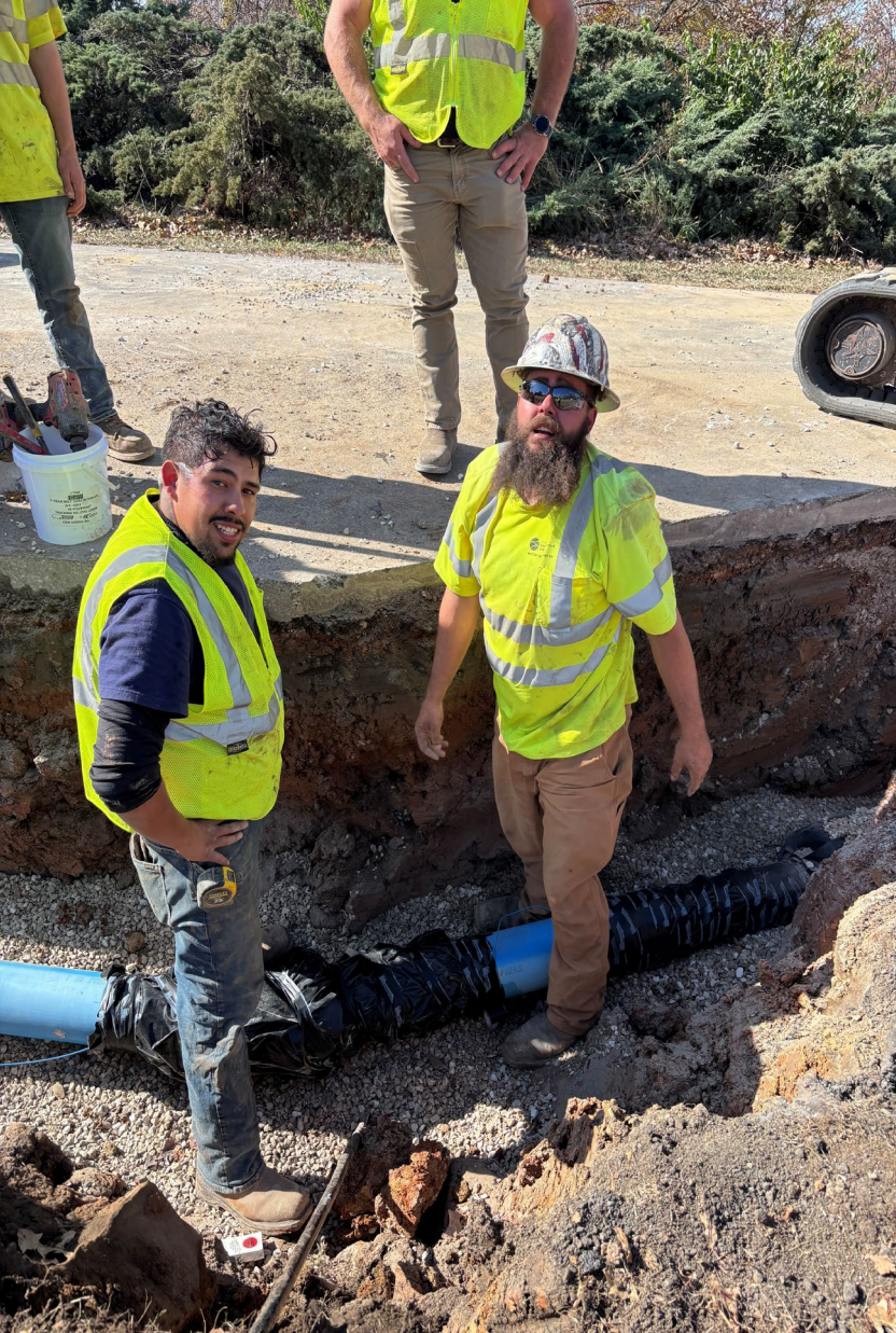
Crew Leader Steven Aldama (right) and new employee Alex Castillo install pipe on Crestwood Drive. Over 2,000 feet of new pipe has been installed so far!
