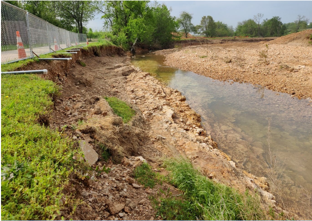
Before and After photos of the erosion threatening the greenway and the restored channel.
