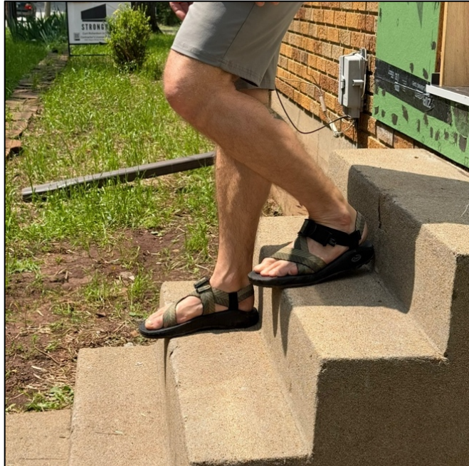
Figure 3. Current out of code stairs at East (kitchen) entrance
