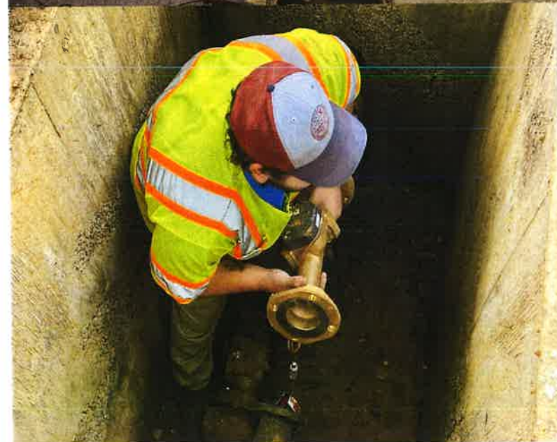
Meter Maintenance Technician Bransen Adams gets ready to install the new meter at Butterfield Trail Village.
