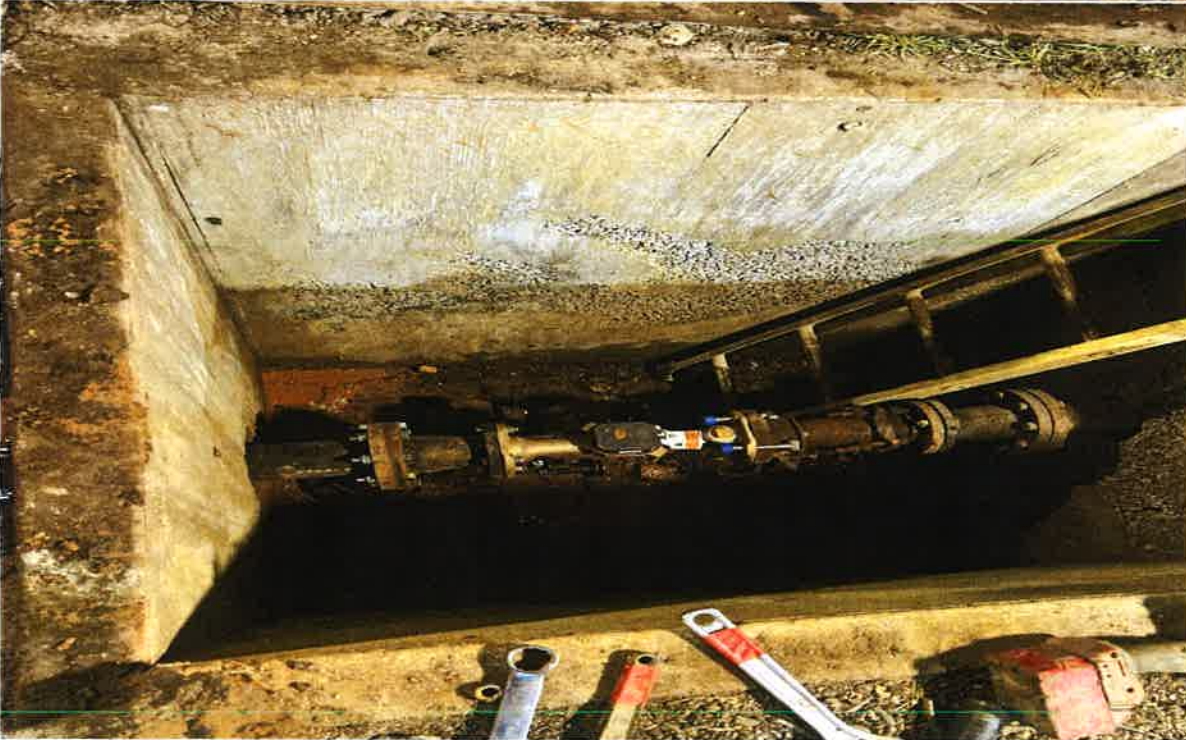
Valve and meter replacement at Butterfield Trail Village completed by Meter Maintenance and Water crews.
