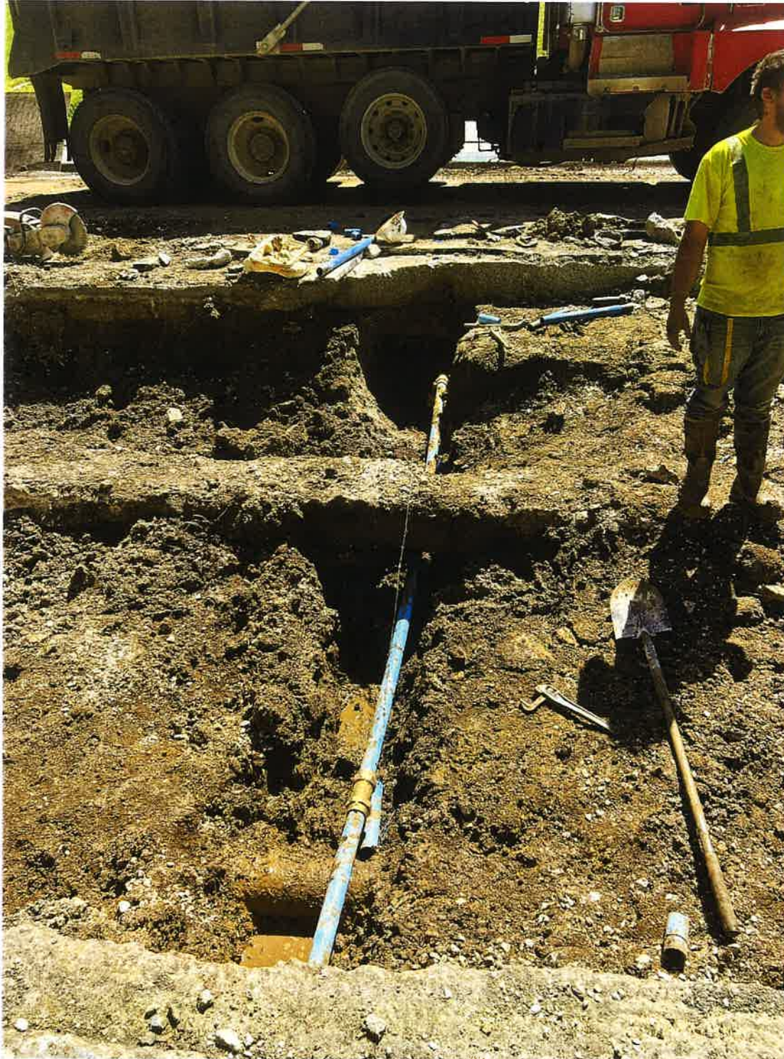
Crew Leader Jacob Standfield and team replace a 2" water service on a road project at the U of A.
