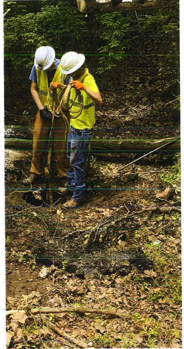
Crew members Michael Coleman (left) and William Bolton (right) work to remove a root ball from a manhole near Crossover Rd.
