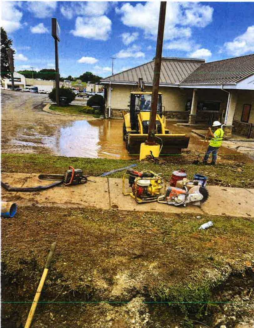
6” AC (asbestos cement) leak on N College Ave.
