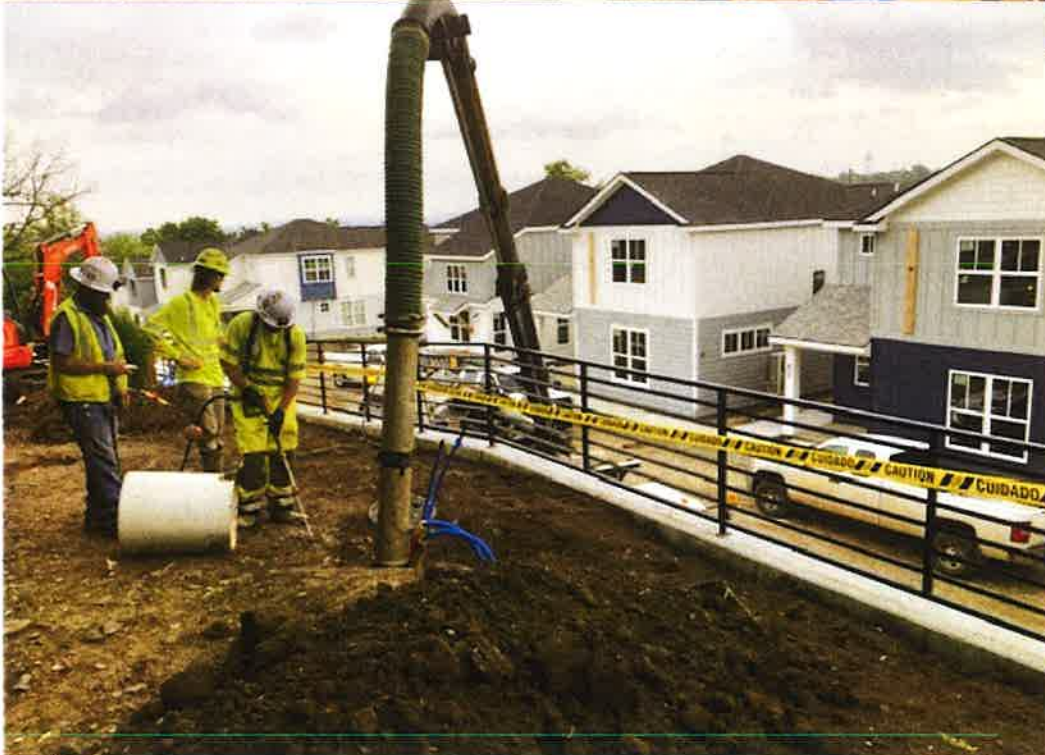
ew Leader Jason McDonner and team -make a new water service tap.
